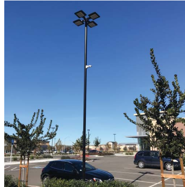
Parking lot lighting shall use energy efficient measures and directed downward
