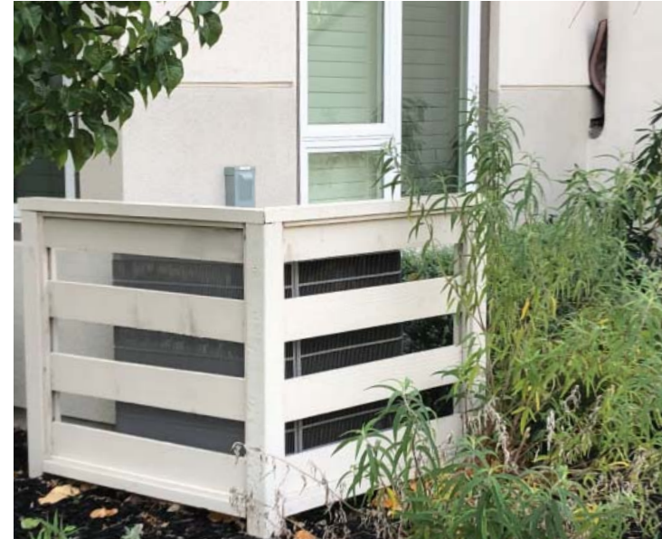
Mechanical equipment shall be screened from public view
