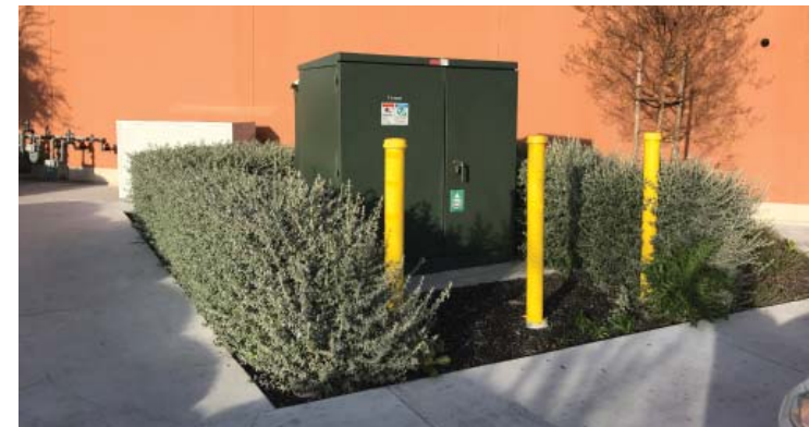
Utility boxes shall be protected from vehicular damage and screened
