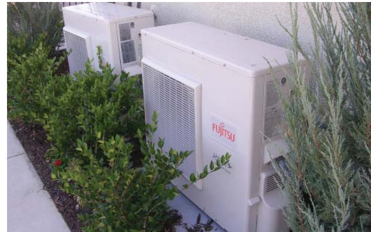
Example of using landscaping as an alternative to shielding mechanical equipment
