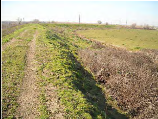
P9-W: View of the levee road and weedy flora on the levee.
