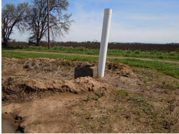
P3-S: View of water well at the southeast corner of Field A.
