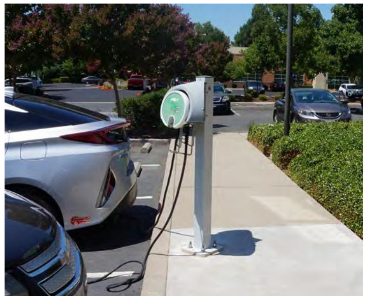
EV charging stations in Elk Grove
