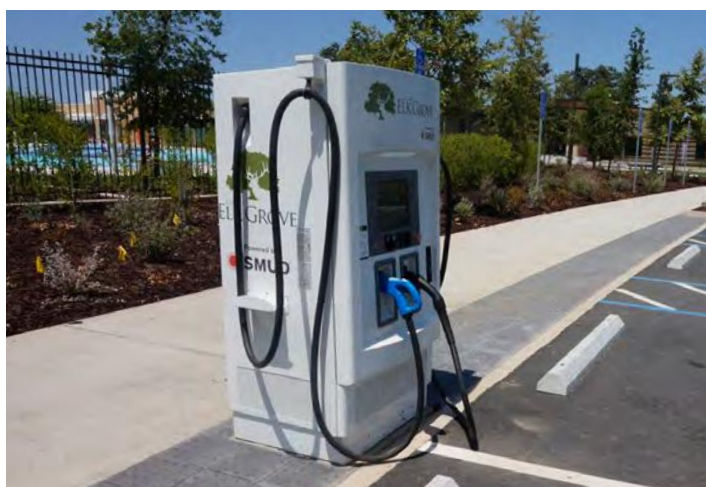
EV charging stations in Elk Grove
