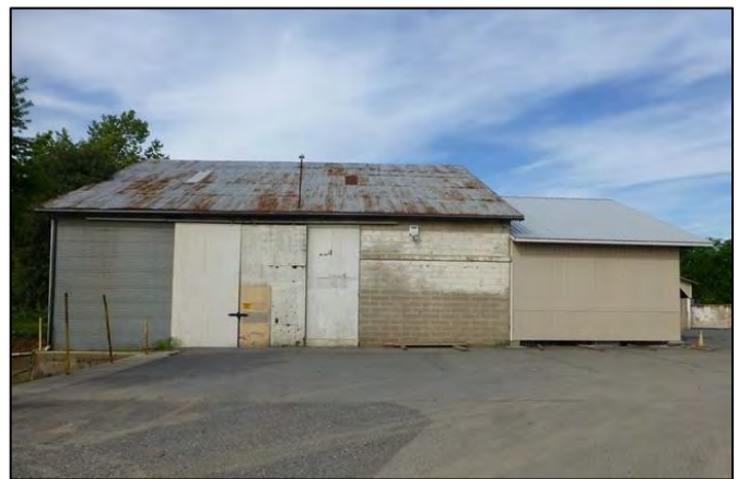
Photograph 14. East elevation of Bldg. 4. Less than half of the building displays its original concrete-block walls. The southern half of the building was rebuilt corrugated metal in 1984
