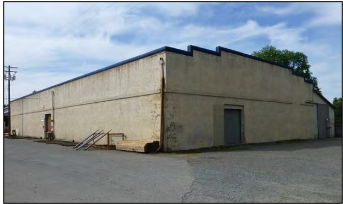
Photograph 13. North & east elevations of Bldg. 5. The original concrete block exterior walls of this building have been altered with a layer of stucco .
