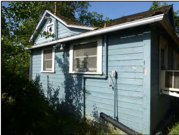
Photograph 10. Closeup of the rear addition at the northeast corner of the building. Camera facing southwest.
