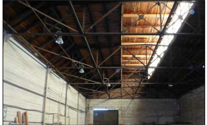
Photograph 10. Bldg. 6, by contrast, displays a steel-truss roof system and no interior posts due to the narrower width of the building.
