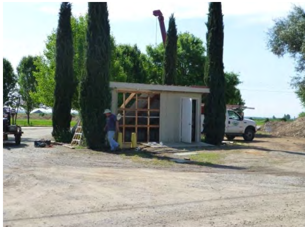
Photograph 5. View southwest of pump house.
