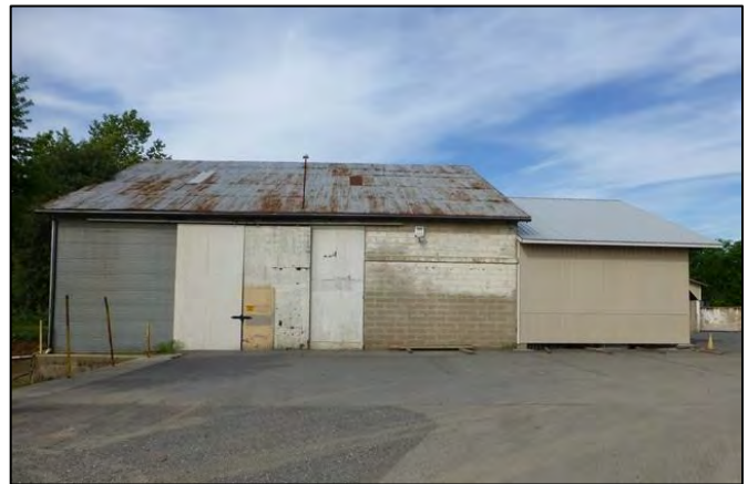
Photograph 14. East elevation of Bldg. 4. Less than half of the building displays its original concrete-block walls. The southern half of the building was rebuilt corrugated metal in 1984
