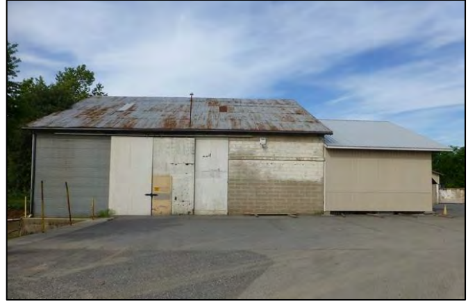
Photograph 12. East elevation of Bldg. 4. Less than half of the building displays its original concrete-block walls. The southern half of the building was rebuilt corrugated metal in 1984
