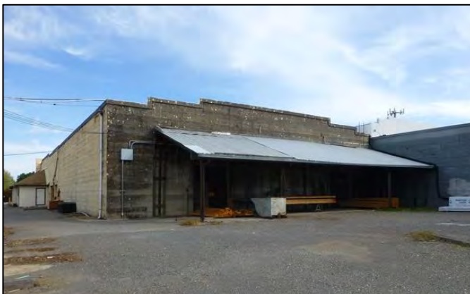
Photograph 3. South and west elevations of Bldg. 5. Note the unpainted, board-formed, reinforced concrete wall, a character-defining feature of this 1915 industrial building.
