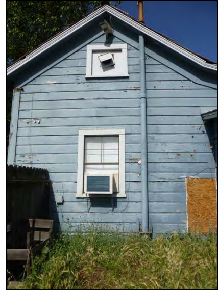
Photograph 9. East elevation of the one-story addition displayed in Photograph 5. Camera facing west.
