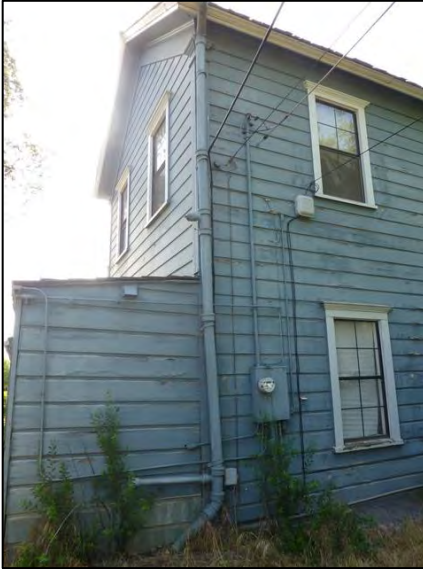
Photograph 7. Northwest corner of the building with a small shed-roof addition on the north elevation of the original massing. Camera facing southeast.
