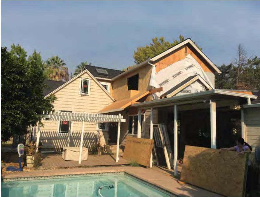
Photograph 4. View northeast of west elevation depicting second-story addition, room addition, and breezeway addition.
