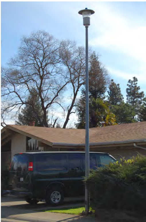
Photograph 7. Representative view of contemporary style street lamp. Taken January 24, 2019.
