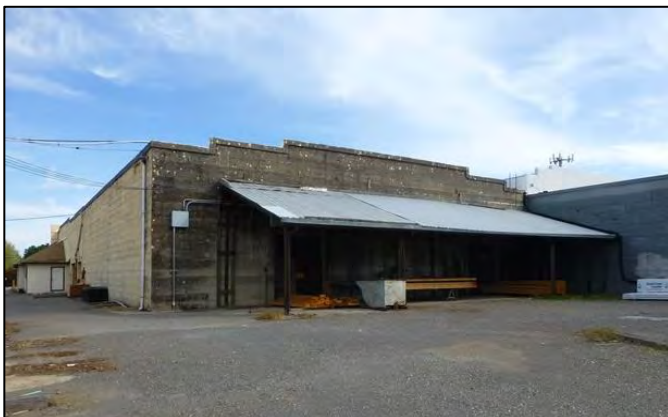
Photograph 3. South and west elevations of Bldg. 5. Note the unpainted, board-formed, reinforced concrete wall, a character-defining feature of this 1915 industrial building.
