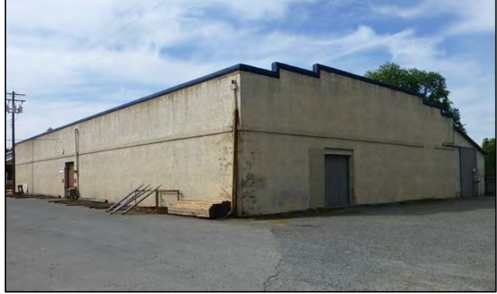
Photograph 16. North & east elevations of Bldg. 5. The original concrete block exterior walls of this building have been altered with a layer of stucco .
