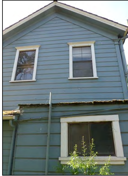
Photograph 8. Closeup of the north elevation of the addition near the northwest corner of the two-story original massing. Camera facing south.
