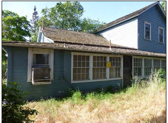
Photograph 6. North façade of the addition affixed to the north elevation of the original two-story massing and an earlier one-story addition. Camera facing southwest.
