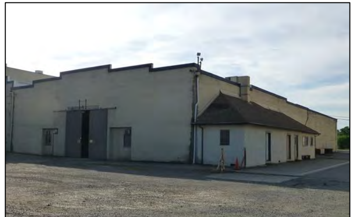
Photograph 2. North and west elevations of Bldg. 5. The half-hipped, truck-scale office appended to the west elevation is not an original feature of the building as constructed in 1915.
