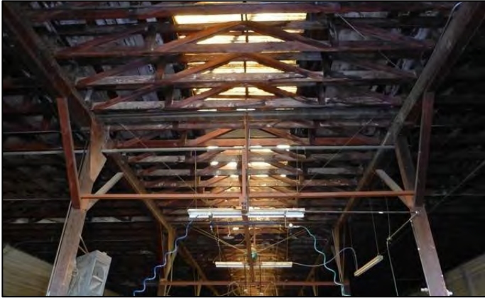
Photograph 9. Bldg. 5. features a timbered -truss roof system supported by knee-braced, square timber posts.
