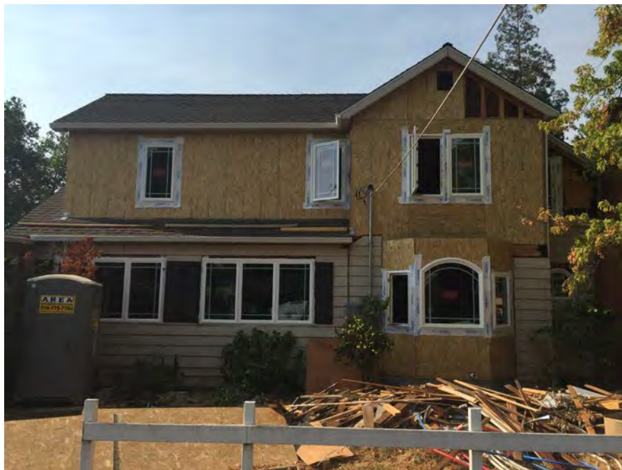
Photograph 3. View south of north elevation depicting large room addition, second-story addition, and new windows.
