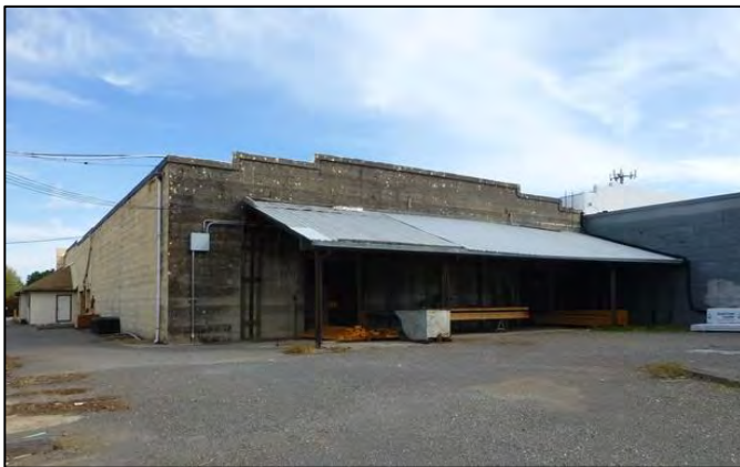
Photograph 4. South and west elevations of Bldg. 5. Note the unpainted, board-formed, reinforced concrete wall, a character-defining feature of this 1915 industrial building.
