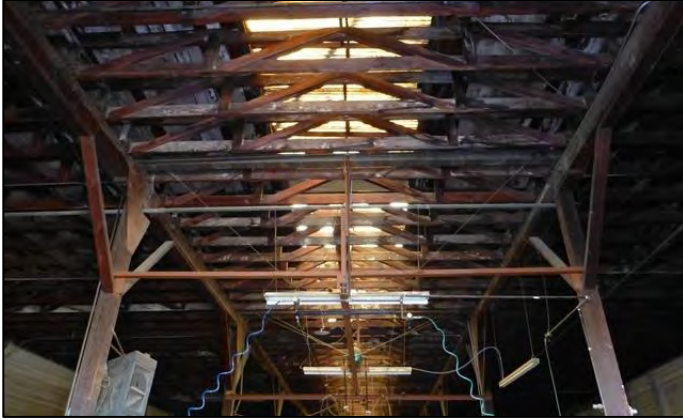
Photograph 5. Bldg. 5. features a timbered -truss roof system supported by knee-braced, square timber posts.
