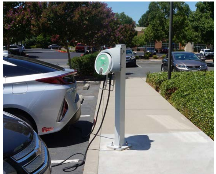
EV charging stations in Elk Grove
