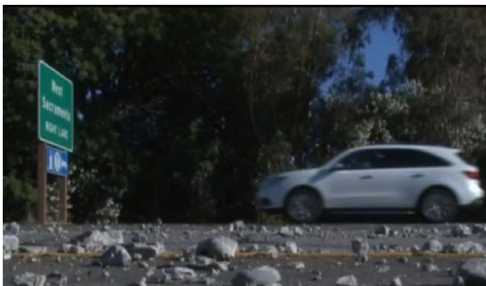
Extreme heat events can result in concrete roadway blowouts in which the pavement expands and can buckle or explode. Highway 50 in West Sacramento experienced blowouts from extreme heat in 2017 (shown above).
