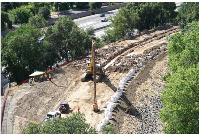
U.S. Army Corps of Engineers construct cutoff wall to reduce seepage and stability issues along the Sacramento River East Levee
