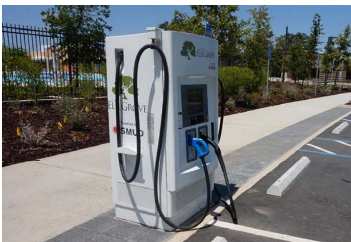
EV charging stations in Elk Grove
