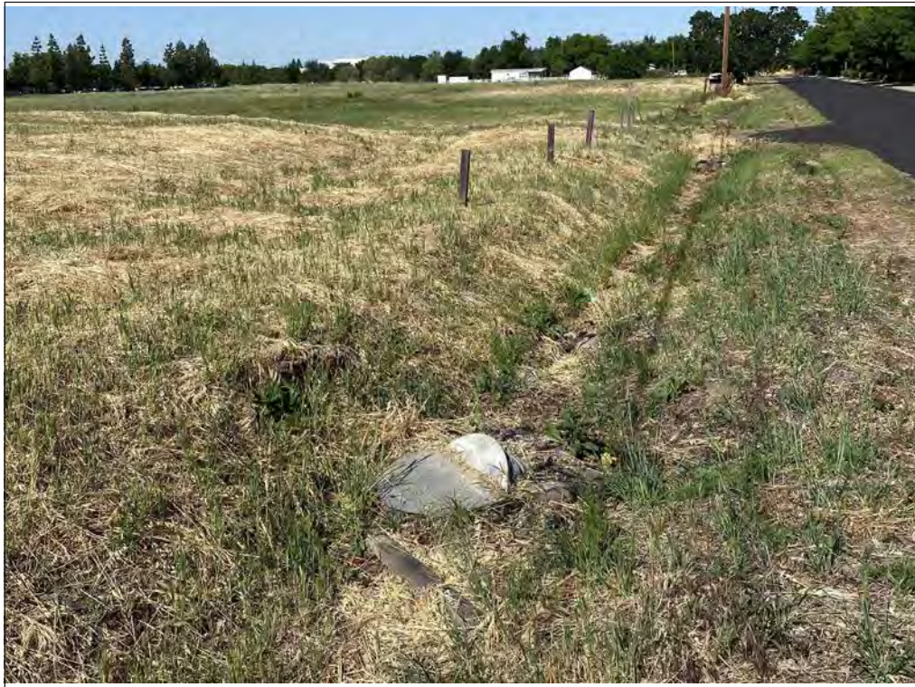
Photo 7. Representative view of the drop inlet culvert that conveys water from D-1 into the stormwater drainage system under Dunisch Road. Photo taken 5/16/2023.
