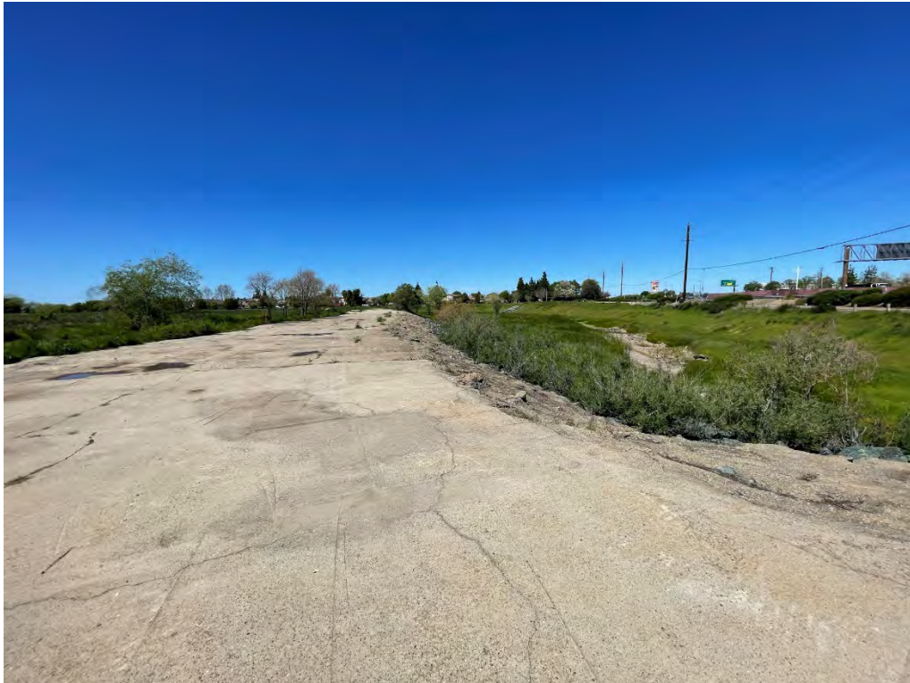
Photo No. 2 View to the northwest of concrete-paved levee from the western portion of the Project Study Area
