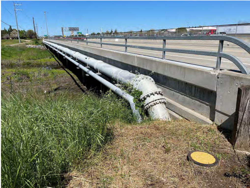
Photo No. 16 Natural gas pipeline along West Stockton Boulevard from the western portion of the Project Study Area
