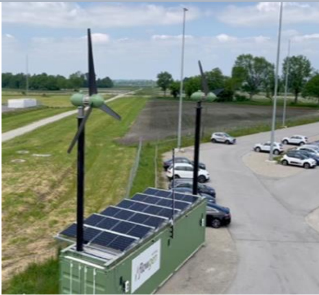
FIGURE 10: 10-KW MICROWIND TURBINES WITH SOLAR AND BUILT-IN BACKUP ENERGY STORAGE
